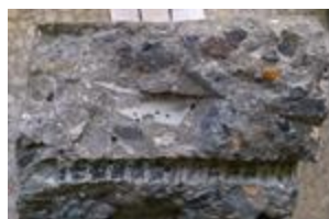
Figure 3: GFRP rebar surface wear
