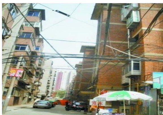
Figure 1 Chaos of the wire in old urban residence
