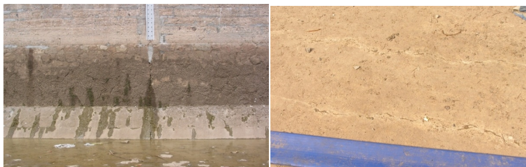
Fig.1 Typical fractures of lock culvert
