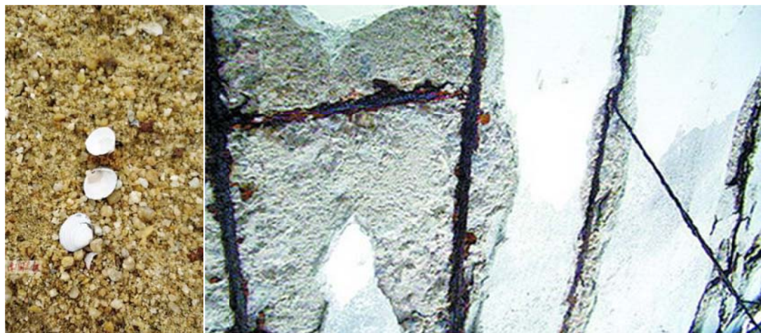
Fig. 2 Sea sand (left) and corrosion of rebar in sea sand-containing concrete (right) [4].
