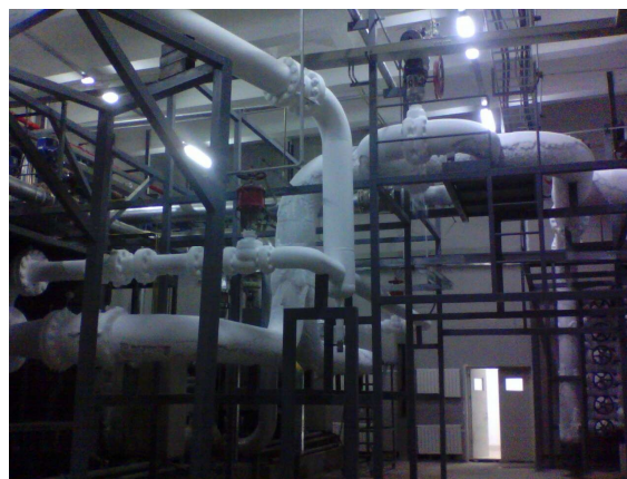
Fig.3 Some zone of the refrigeration subsystem
