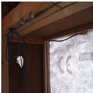
Figure 7. The location of the sensors in the construction.
