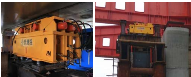
FIGURE IV. IL DEVICE, IN ORANGE, TOGETHER WITH HEIGHT ADJUSTMENT JACKS, IN RED, ARE ASSEMBLED IN THE BOTTOM OF THE SUPPORTING PLATFORMS TO ADJUST THE HEIGHT OF LAUNCHING PLATFORMS
