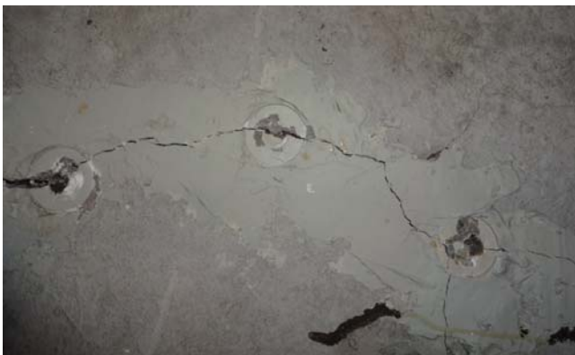
FIGURE VI. EVENTUALLY DESTROY FORM OF REINFORCING MIDDLE MAIN CRACK
