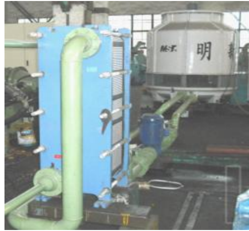
Fig.4. Water cooling tower, pump and heat exchanger
