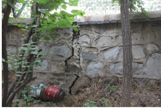
Fig.4 The ground fissure of painteryard
