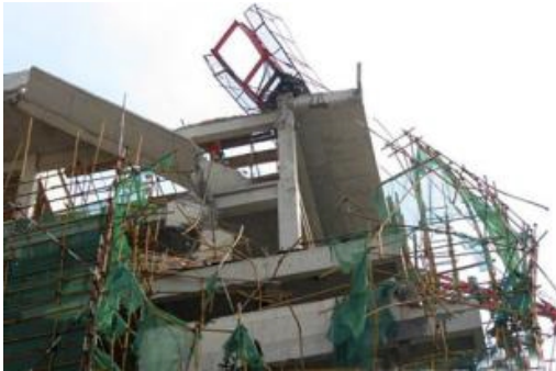
The counterweight of tower crane destroyed the building
