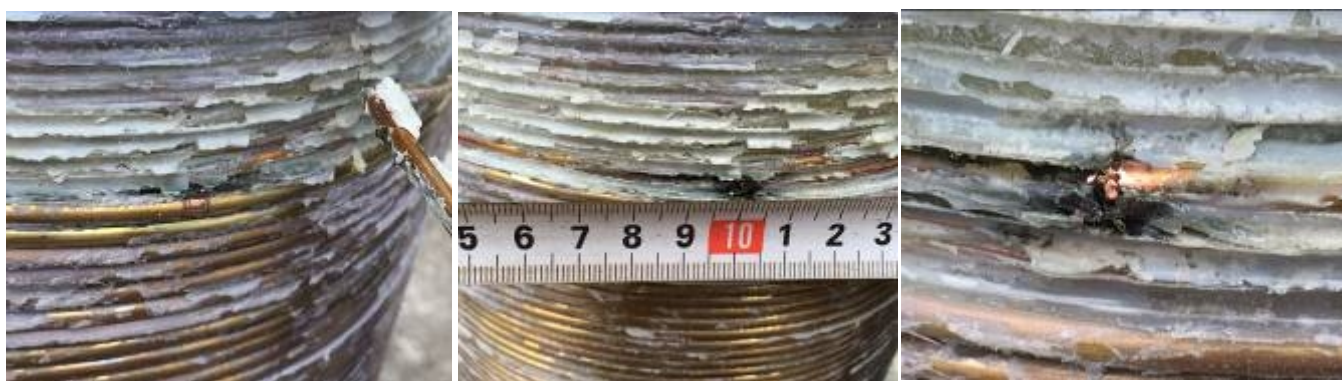
Fig.5 Short circuit position and discharge trace
