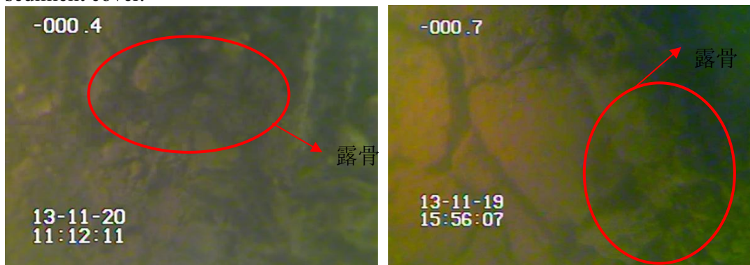
Fig.2 Right 15-1# pile foundation, uneven concrete
