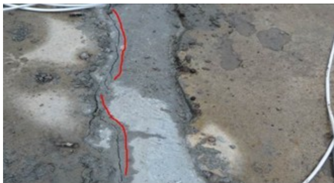
Fig. 5 The crack of shear key in the topping when load reaches 80.6t
