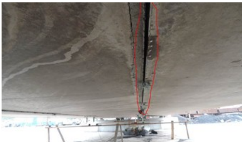
Fig. 6 Failure of the hinge joint
