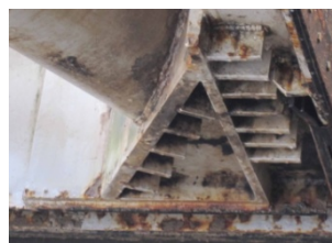
Fig.2 A sluice connection
