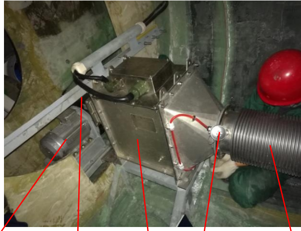
Electrical machine Air blower Heater PT100 Ventilation pipe
