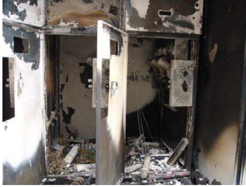
Fig.1 The pollution flashover of user switchgear
