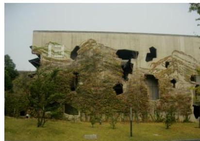
Fig. 5. Long view of holes in outer wall on Xiangshan campus.
