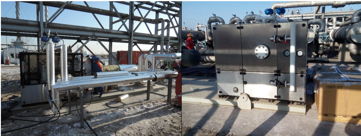
Figure 2. On-site pictures of online cleaning system
