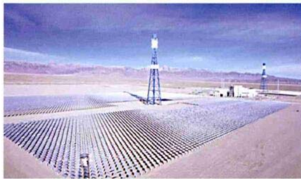
Fig. 2 the first phase of the 50MW tower solar power station in Delingha, Qinghai Province
