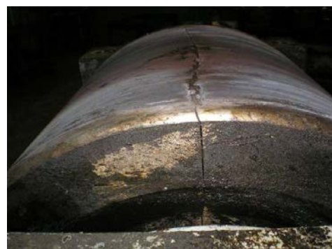
Fig.2. A crack extending inward
