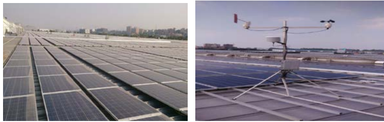
Fig 2. The rooftop PV power plant
