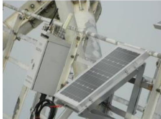
Figure 7 Aeolian vibration monitoring base station.
