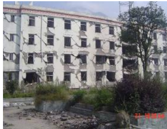
Fig 6 Dormitory of Yingxiu middle school suffered "X" shear cracks
