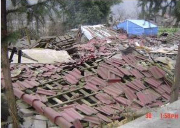
Fig.1 Complete collapse of brick-wood structure
