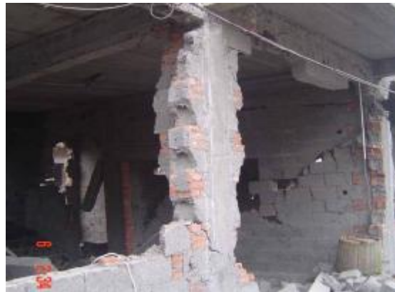
Fig 4 Loading failure of constructional column
