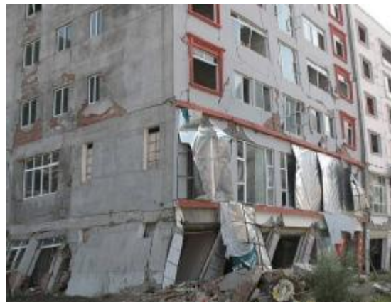
Fig 8 Brick-concrete structure of bottom frame with serious damage
