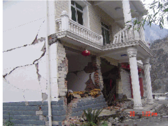
Fig 2 Earthquake disaster characteristics of brick-concrete structure
