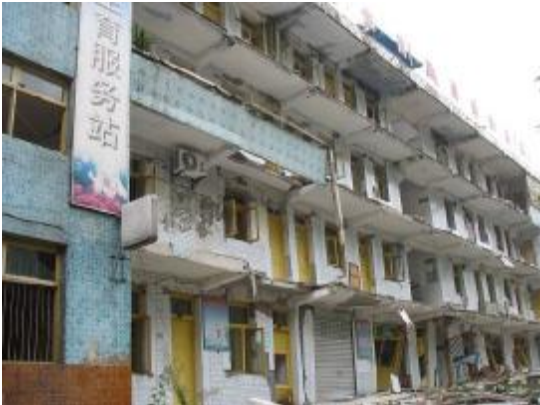
Fig 3 Brick fence in outside corridor of office building collapsed
