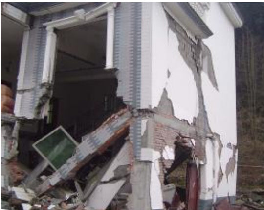
Fig 5 Loading failure of ring beam
