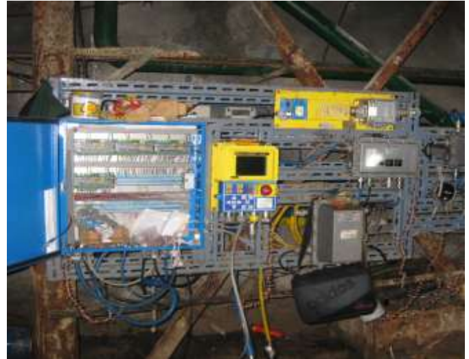
Fig. 13. Becker pumping equipment automation
