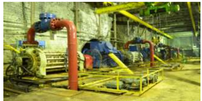
Fig. 1. Pump chamber of the main mine drainage system at the Udachny mine
