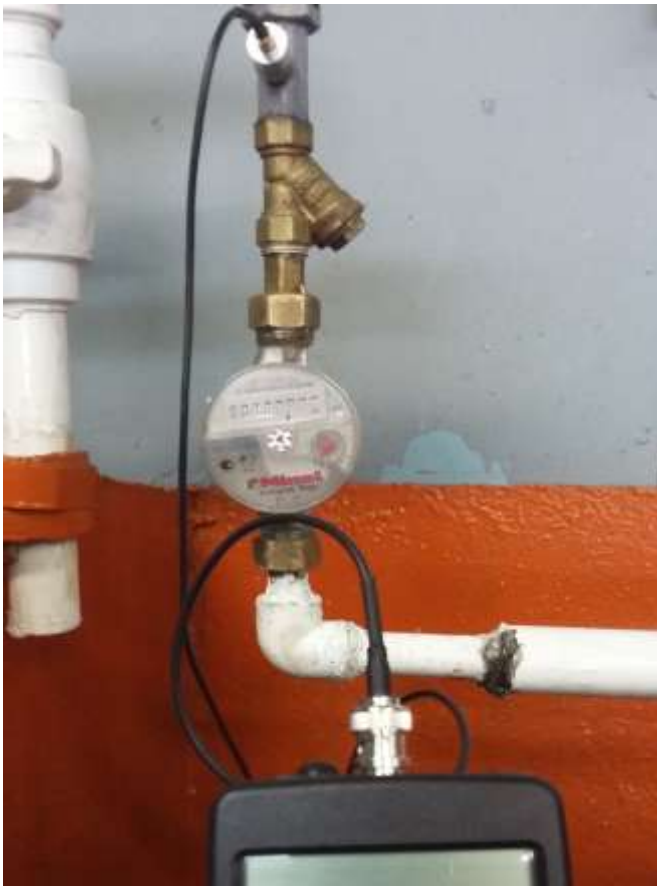
Fig. 18. Research of the RMS values of the pipe vibration velocity
