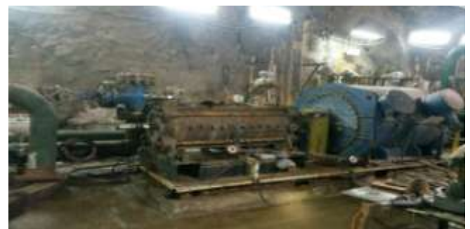
Fig. 2. Pump chamber of the main mine drainage system at the Mir mine
