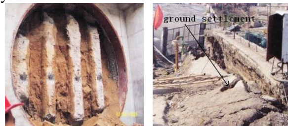
Figure 1. Diaphragm wall breaking and ground surface collapse of a shield tunnel end soil
