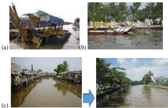
Fig 4. Maintenance of rivers and river normalization, (a) river dredging using Biyoko boats, (b) river cleansing using Sapu-Sapu boats, (c) normalization of JafriZam-Zam River (Photo by DSDAD of Banjarmasin, 2016).
