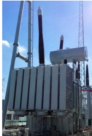
Fig. 2 500kV Series Transformer
