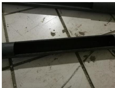
Fig.2 Local damaged member
