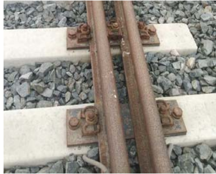
Fig.3 The image of rail fasteners
