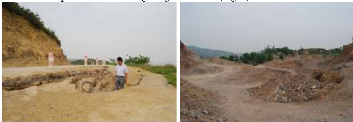
Figure 4. Finite Underground mining of clay minerals leads to the collapse of highway subgrade and damage of natural landscape
