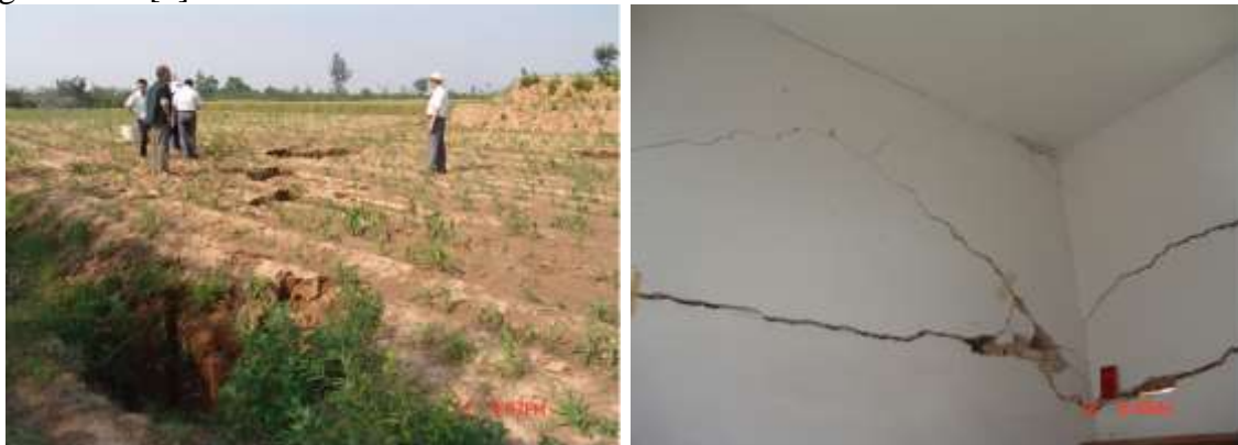
Figure 2. Finite Subsidence and house cracking caused by coal mining
